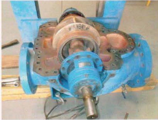
Split case Pump(Chilled water)
